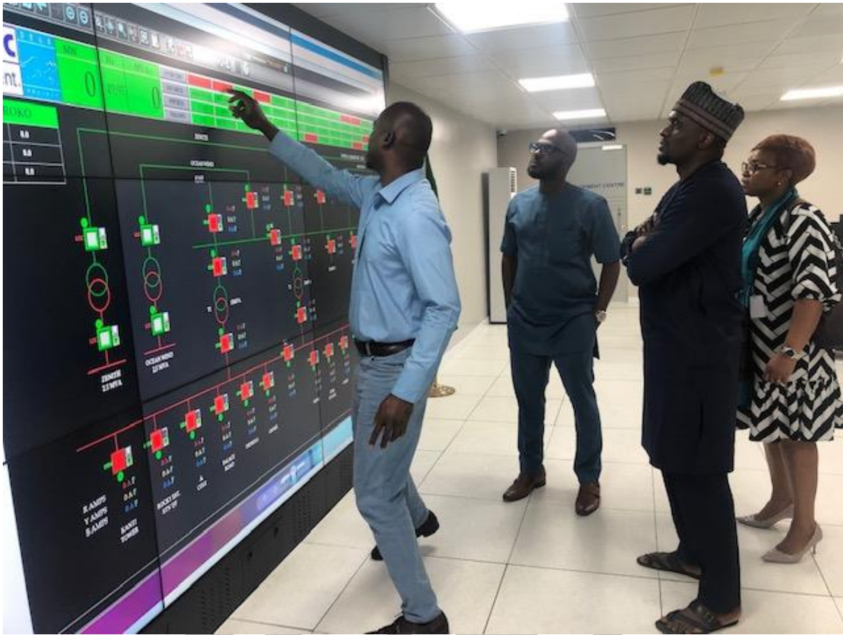
Figure 8: SCADA room showing real-time network monitoring
